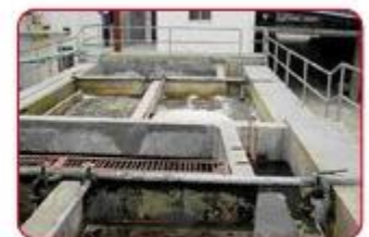
Sewage tank water level measurement
